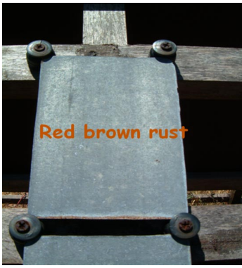
Figure 6. Galvanized Fe sample at site S1.
